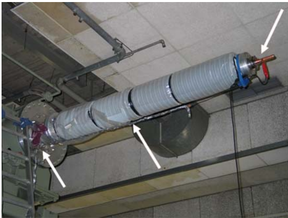
Fig. 3: Measurement connection on bushing stem and ground connection with aluminium braid on a 400 kV bushing
